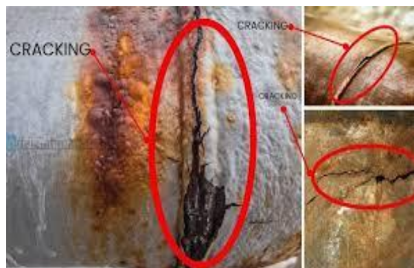
Figure: Stress Corrosion
