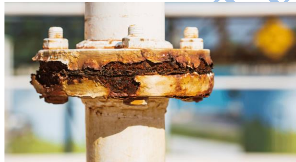
Figure: Galvanic Corrosion
