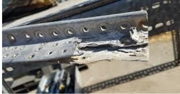
Figure: Intergranular Corrosion
