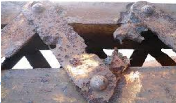
Figure: Pitting Corrosion
