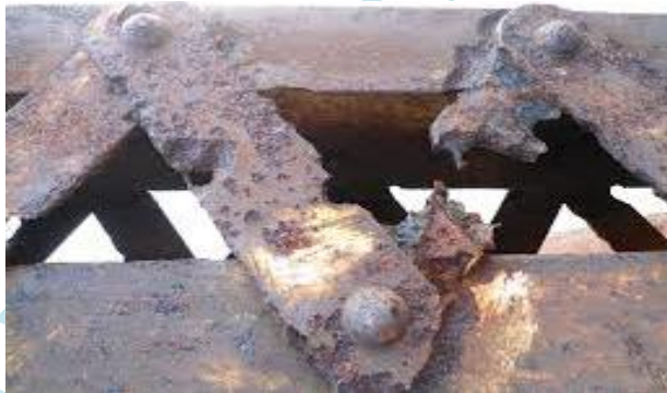
Figure: Pitting Corrosion
