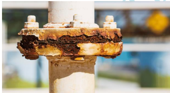
Figure: Galvanic Corrosion
