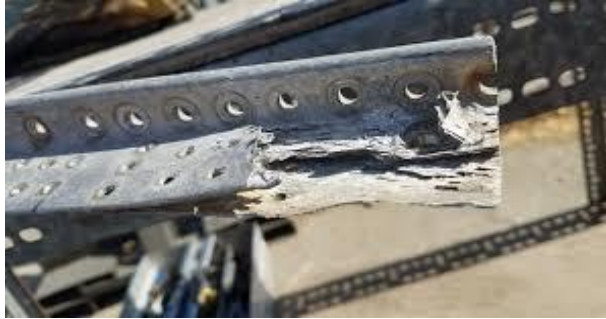
Figure: Intergranular Corrosion
